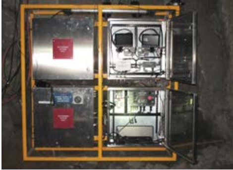
Sub level Teleremote control cabinet
