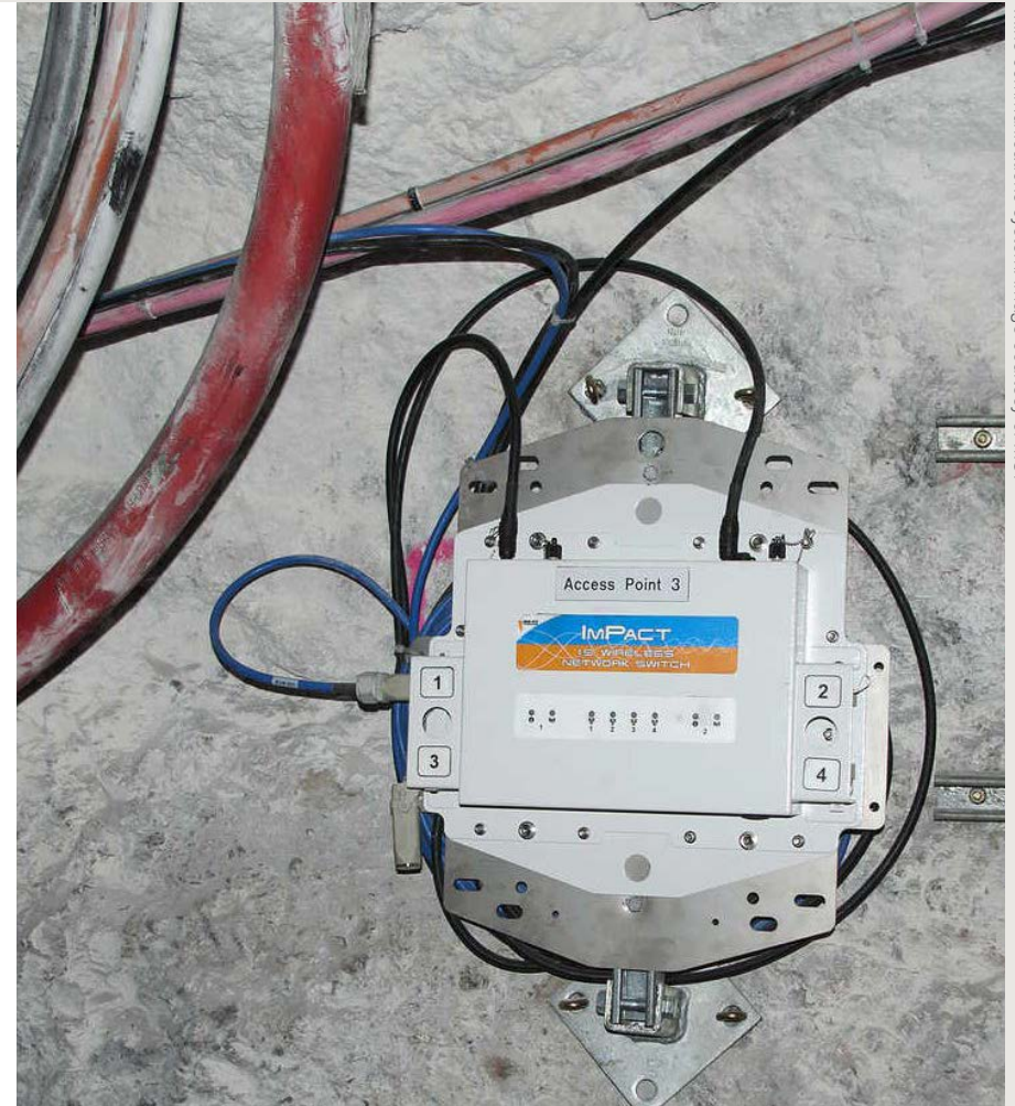
Mine communications system. Image courtesy of MST
